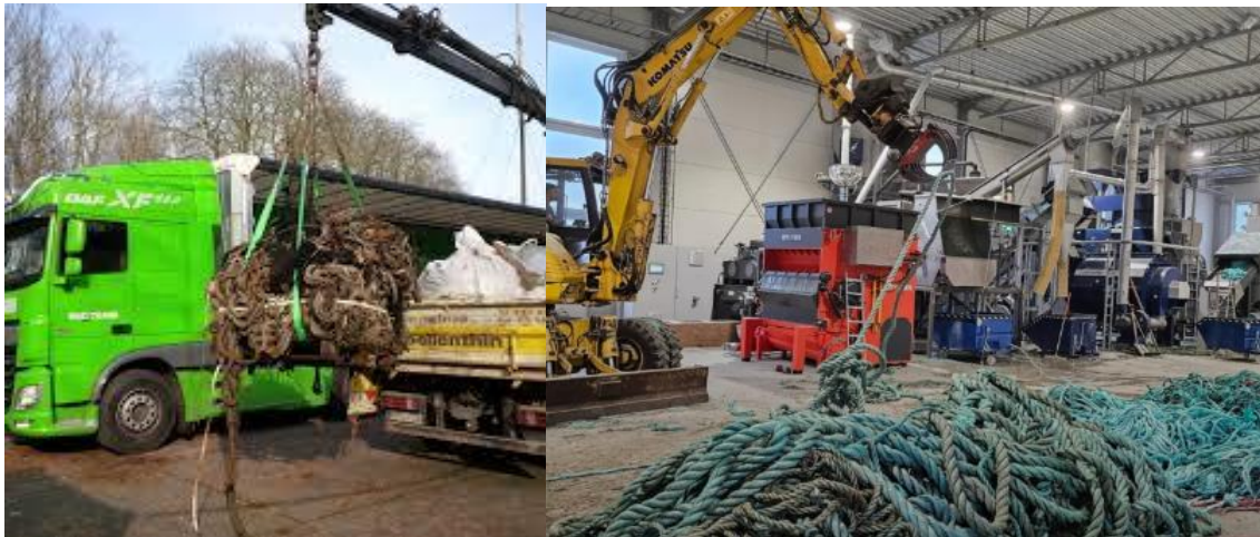
Figure 14. EOL FG heavy duty truck loading, sorting infrastructure and backhoe loader used for handling
